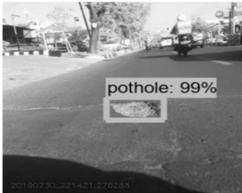
Figure 8 Pothole detection result (Rasyid et al., 2019).
